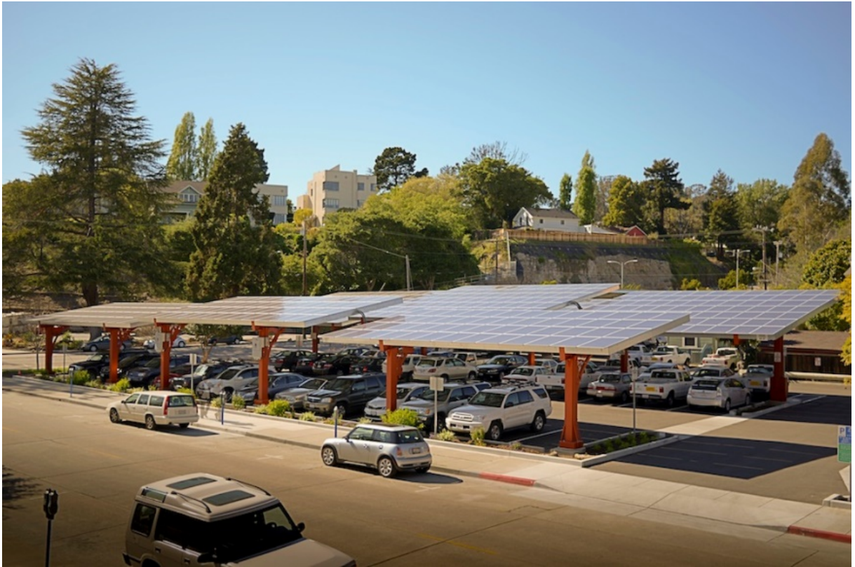
FIGURE 1.3: Solar parking lot in Santa Cruz, United States.
